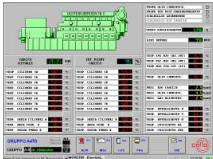
Each of the eight generating plants is monitored by an equal number of graphic synoptics like the one shown in the figure.
