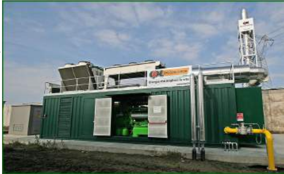
One of the 4 Jenbacher motors, situated in a container purposely designed to house all the process components needed for efficient system management.
