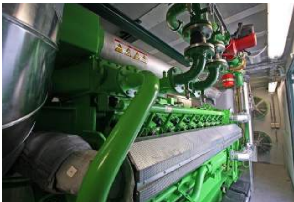
The four cogeneration motors are injected with the gas produced by the biomass to produce a total of 4 Mwe of electric power with zero CO2 emissions.
