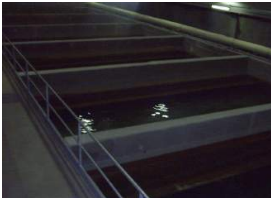
Detail about one of the basins used for the water purification system.
