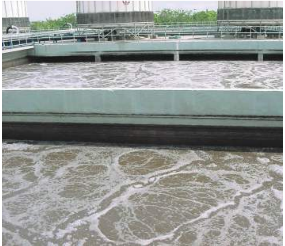
3. The industrial wastewater treatment plants are essential to managing water cycling properly in accordance with the laws to protect the environment in which we live.
