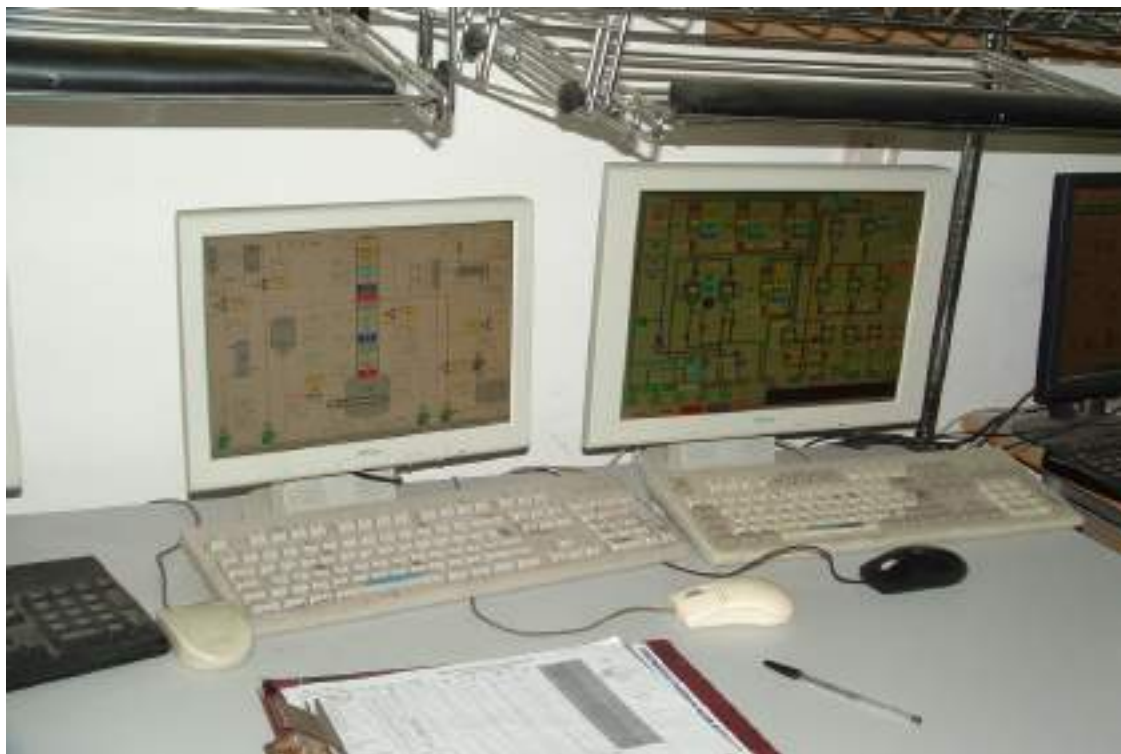
The Biodiesel plant Control Room. The plant workers can control the whole process using the redundant Movicon supervision workstations.
