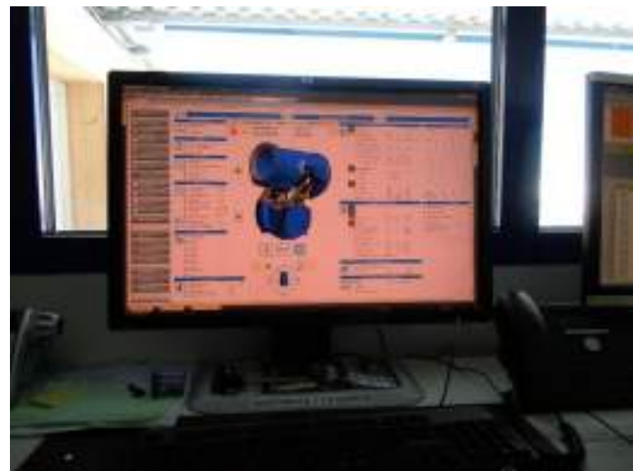
One of the Movicon supervision system control station terminals at St. Moritz - Engadin
