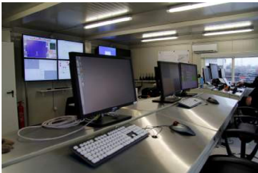
4. Control Room with Movicon 11 screens displayed on video wall
