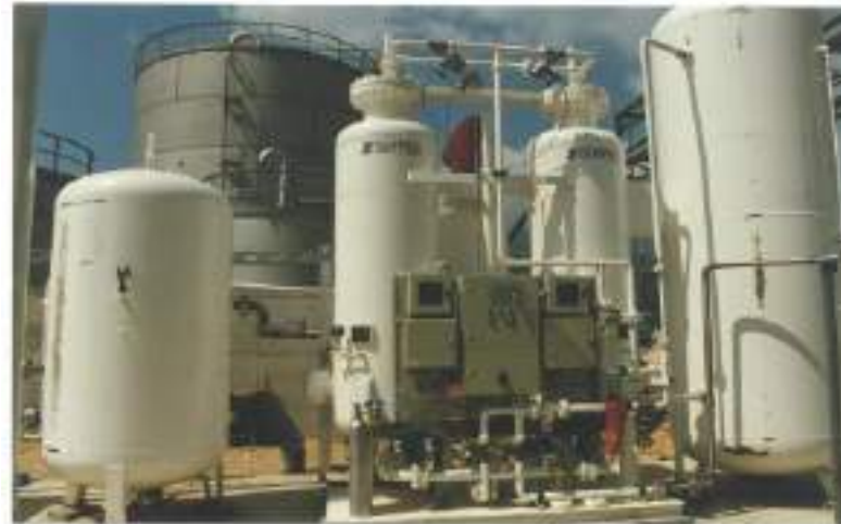
One of the self-production plants of the Sapio group, which has stations scattered throughout Italy.
