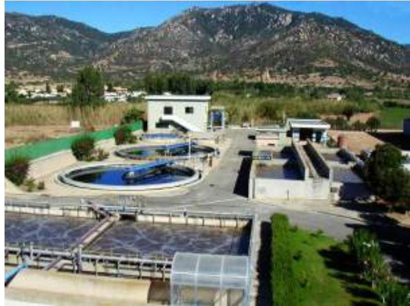
The wastewater treatment process monitored and remote controlled by a system designed by Anova Srl from Naples.
